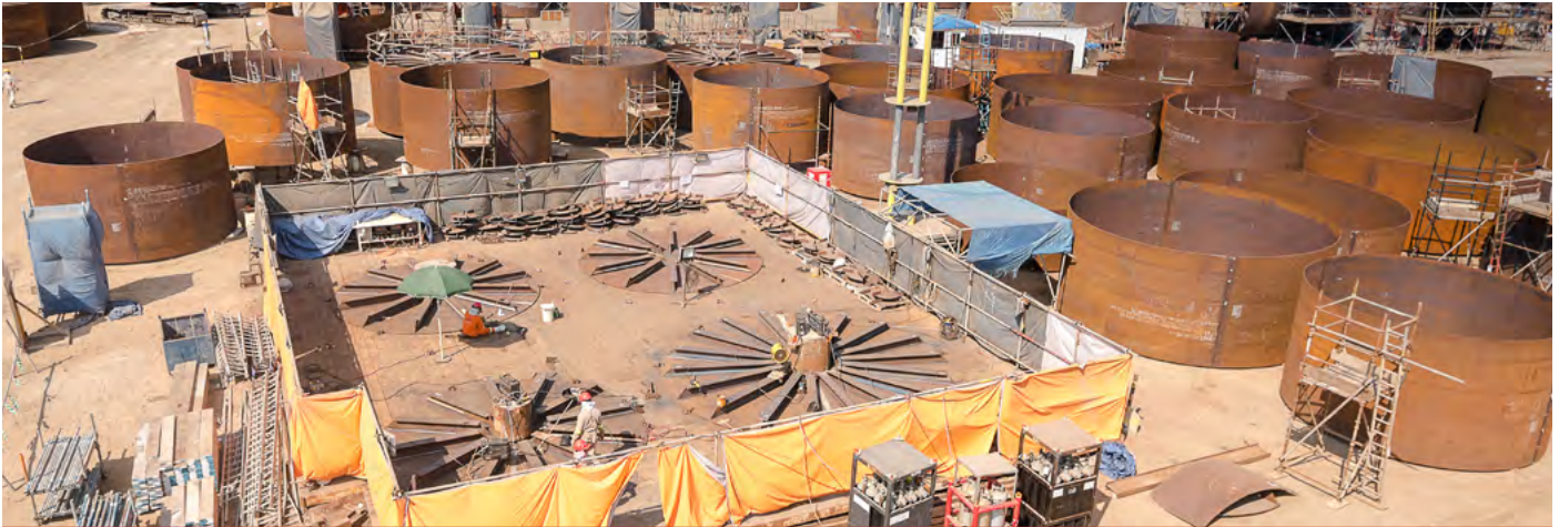
Fabrication of suction piles and buoyancy tanks are progressing on schedule for the Kaombo Project
