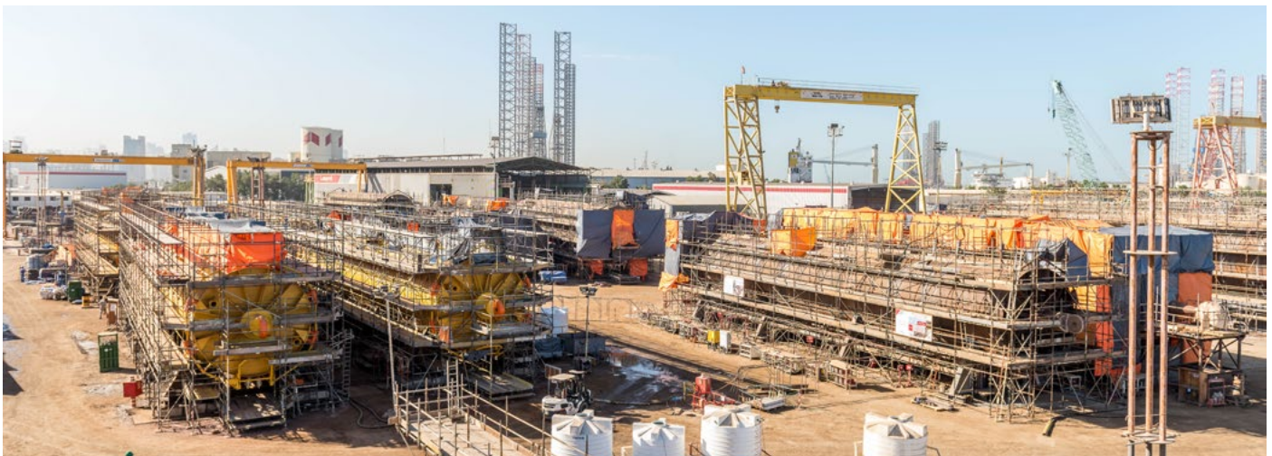
The Kaombo project team celebrated progress and reaching two million manhours without a DAFWC in December 2016
